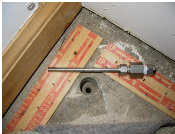
Figure 1: Assembled sub-slab port ready for installation
